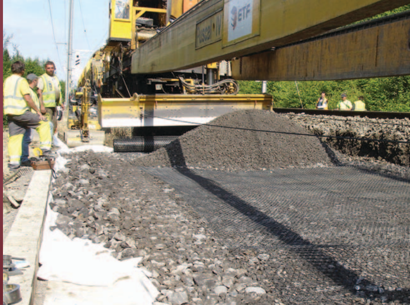
Tensar® TriAx® geogrids installed under the granular sub-ballast layer to increase bearing capacity (Belgium).
