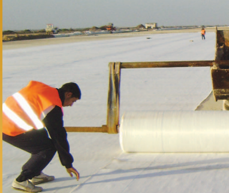
Tensar® Basetex™ geotextile installation at Oran airport in Algeria providing cost-effective installation and offering permanent high strength reinforcement below the fill layer.
