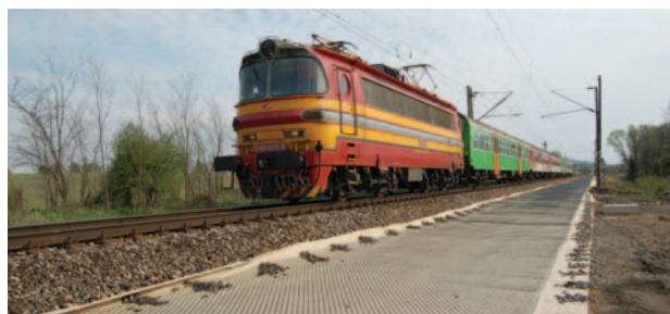
Track reconstruction over low bearing capacity subgrade soils using Tensar® TriAx® mechanically stabilised sub-ballast. (Bratislava, Slovakia).
