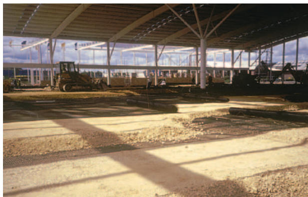
LTP to support a concrete ground floor slab beneath a steel portal frame building (UK).
