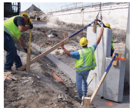
TensarTech Ares panels are laid on a concrete levelling pad and subsequent lifts of panels are dry laid.
